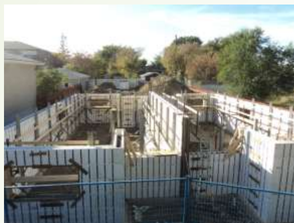
The completed ARXX ICF Course work is now ready for pouring and the foundation for the duplex will be set!
