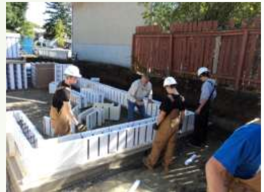
HCAP, Habitat finishing up the first "course" by assembling the formations, laying the rebar, zip tying, and then next course!
